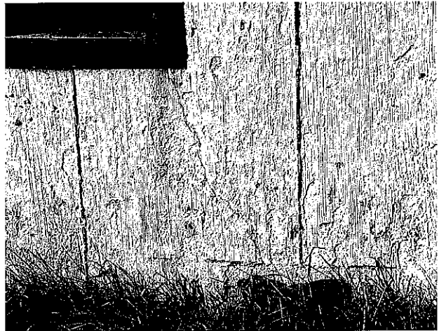
10 – Vertical crack at lower corner of south window on east side. This is a shrinkage crack.
